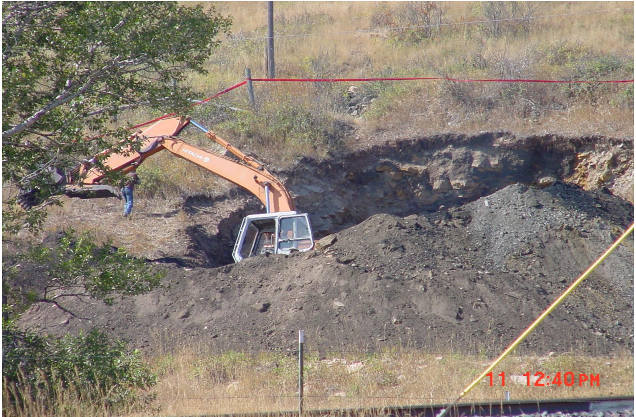
Figure 24. Excavating cover material for access to old mine adit, Anaconda Coal Mine.
