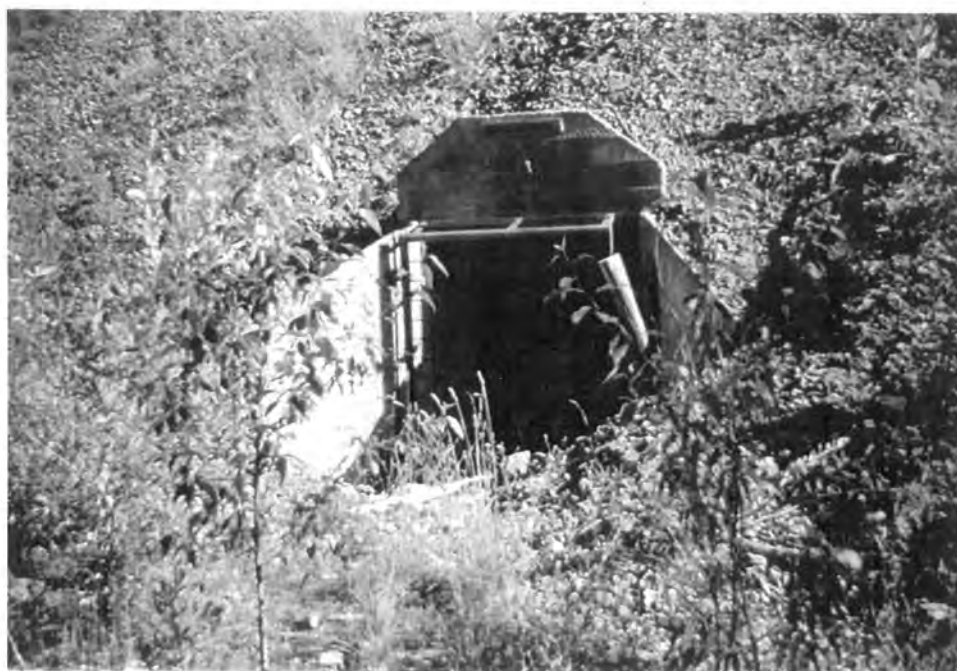
Figure 6.26 A gate across the adit entrance at the Hidden Treasure mine has been vandalized so that it is now possible to crawl into the mine workings.
