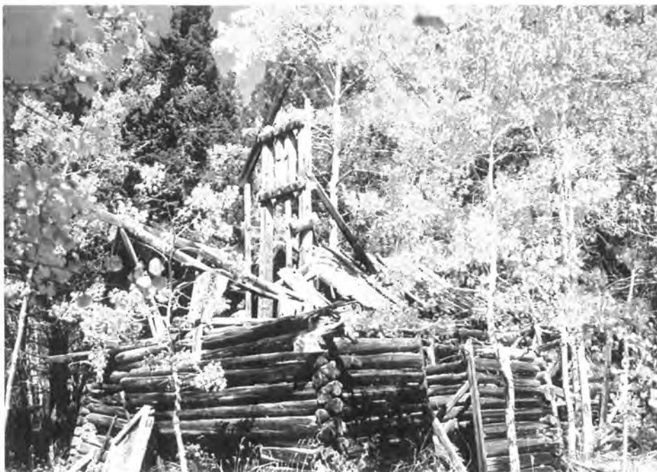
Figure 6.7 Hoist house/mine shop may cover an open, 100' shaft.
