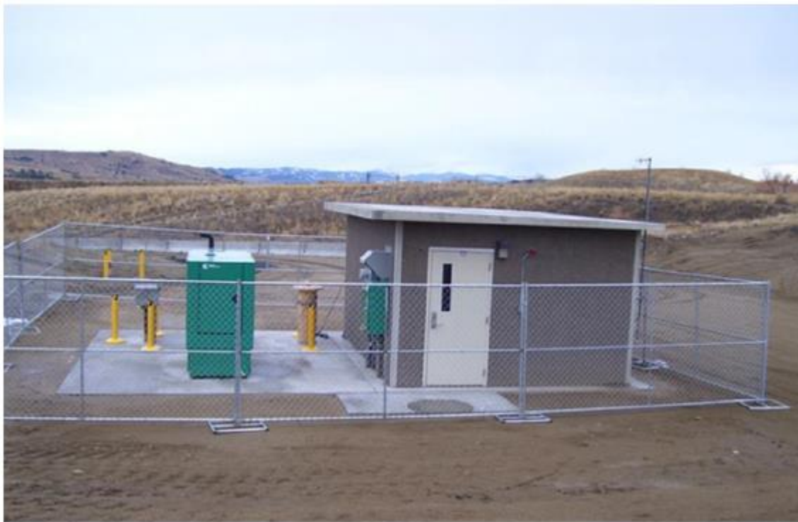
Figure 4-5. West Camp pump station upon completion in 2011.
