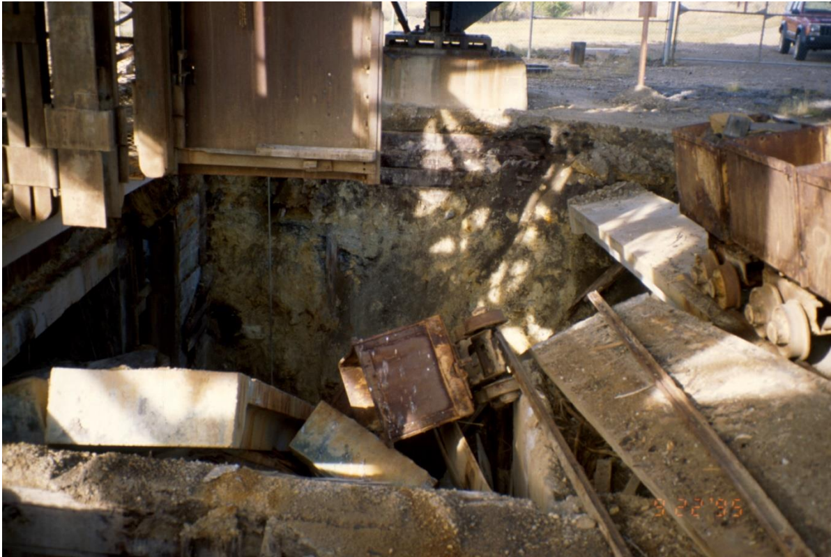
Figure 3-20. Mine shaft and adjacent area collapse at the Belmont Mine.
