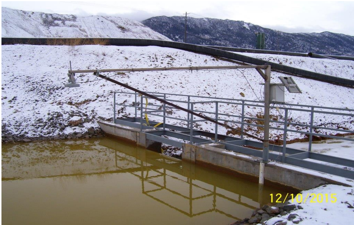
Figure 3-27. Radar system installation at the Horseshoe Bend weir monitoring station.
