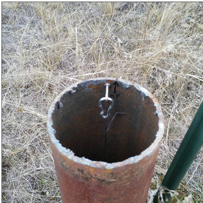
Figure 4.1. Suspended cord installation with eye bolt, carabiner clip, and Kevlar cord. The bolt-on well cover is removed from the well in this photo. Note sharp metal edge along the top of the casing.
