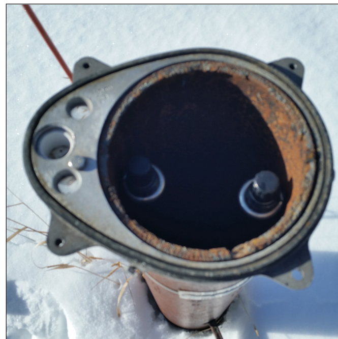
Figure 4.4. Direct read cables from a barometric pressure transducer and a non-vented pressure transducer are affixed to eye bolts. The bolt-on well cover is removed from the well in this photo.
