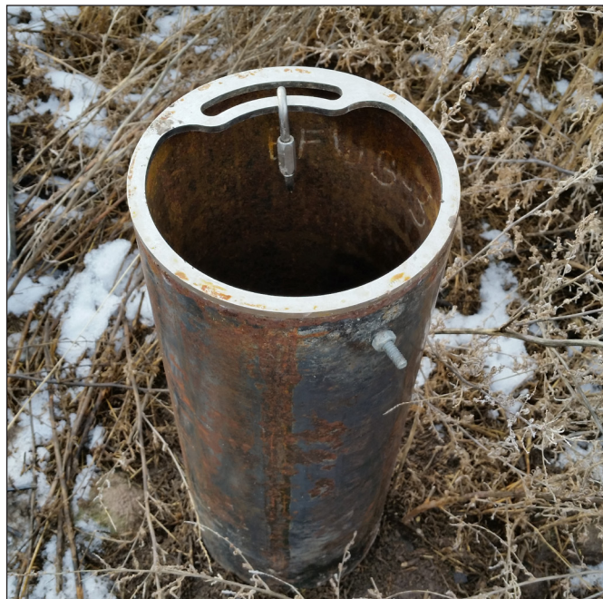
Figure 4.2. Suspended cord installation using well collar with attachment point. The bolt-on well cover is removed from the well in this photo.
