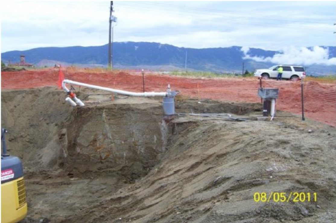
Figure 4-3. West Camp pumping well, discharge line, and monitoring well exposed during 2011 construction activities.
