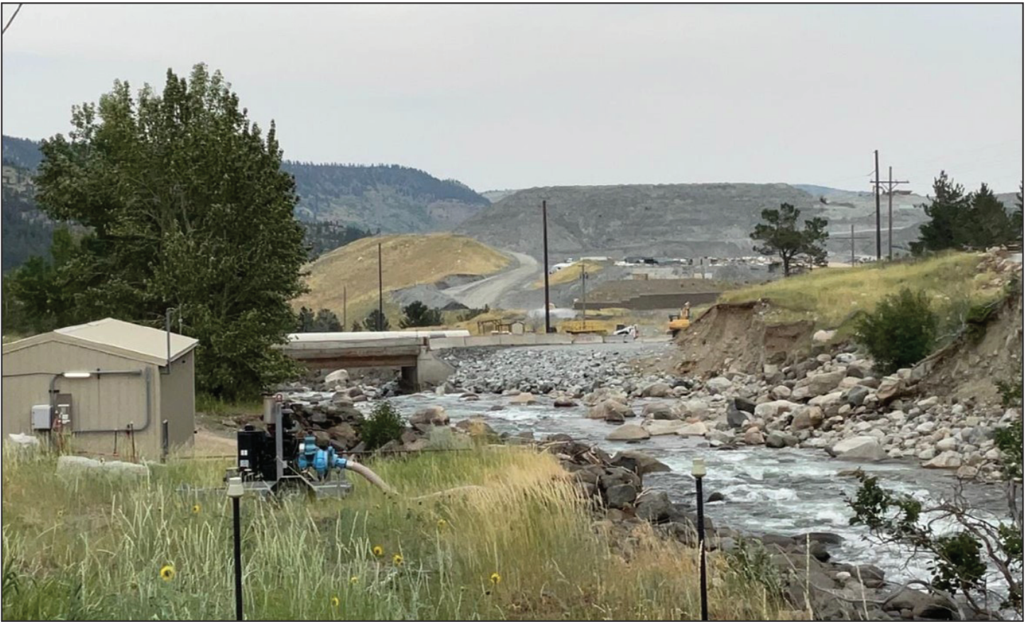
Figure 4. From August 2022 site inspection, the bridge repair at the Stillwater Mine nearing completion following the June flood.
