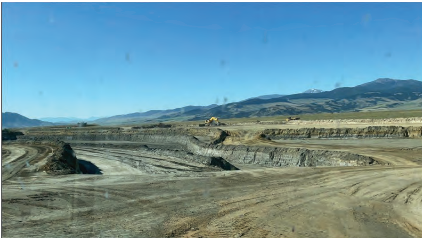
Figure 3. Excavation of the tailings from TSF-1 at the Golden Sunlight Mine. The existing reclamation soil cap being salvaged for future use, following the removal and reprocessing of waste from the unlined facility.
