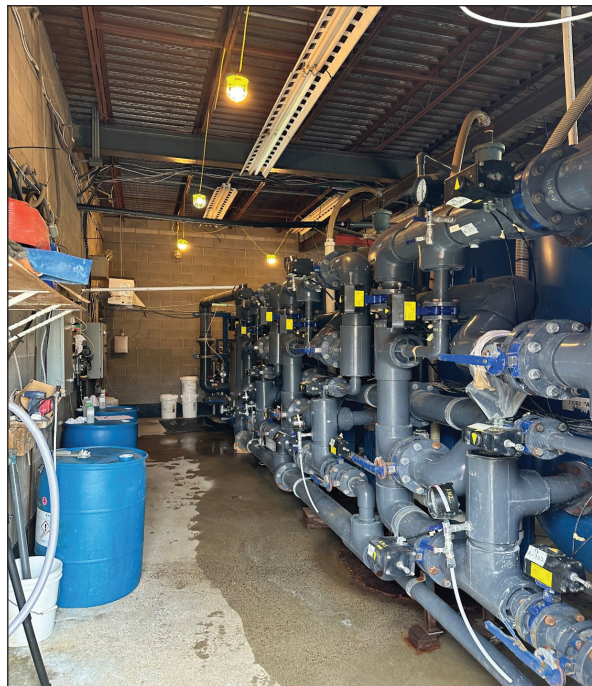
Figure 3-6. Inside the Beal Mountain Water Treatment plant.
