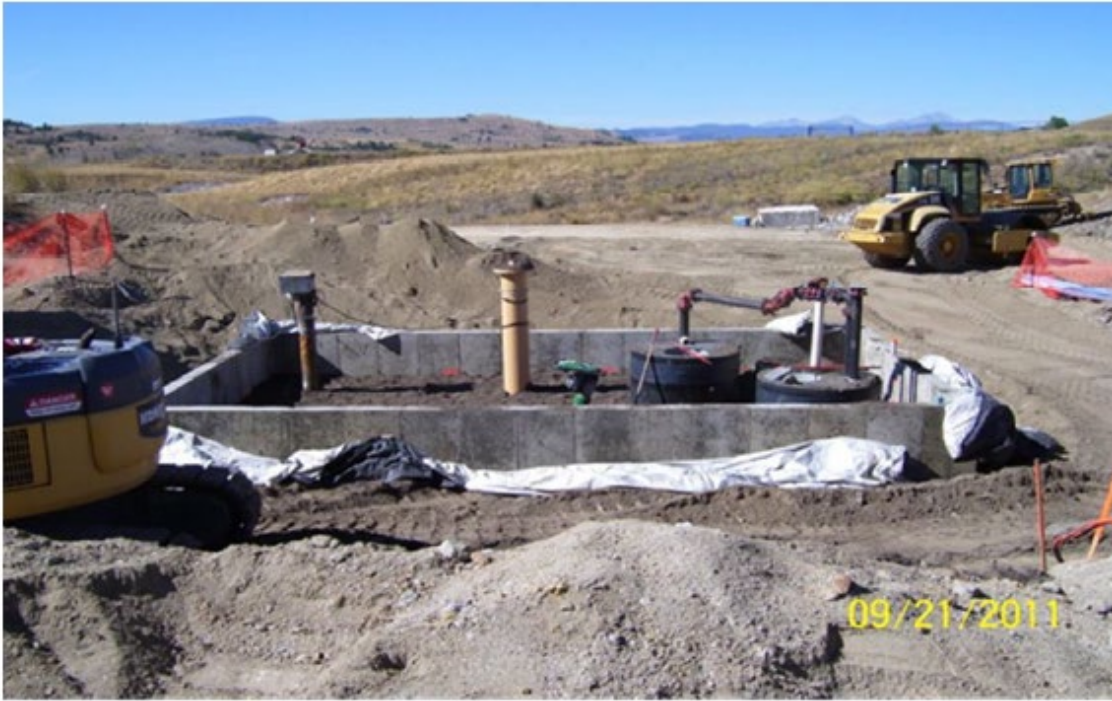
Figure 4-4. West Camp construction activities showing a new pump station foundation and infrastructure improvements surrounding the pumping well and discharge line.
