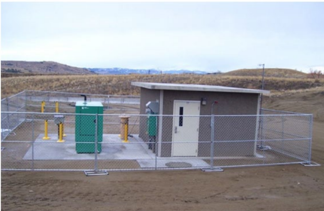
Figure 4-5. West Camp pump station upon completion in 2011.
