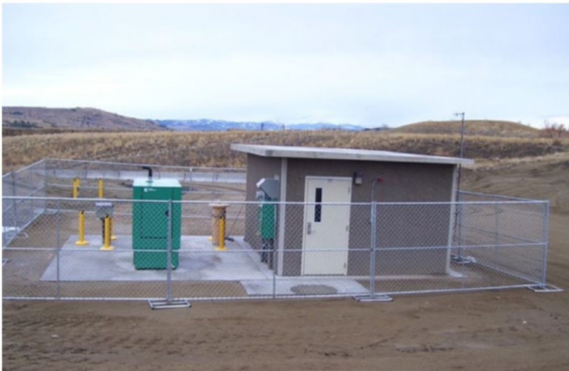
Figure 4-5. West Camp pump station upon completion in 2011.
