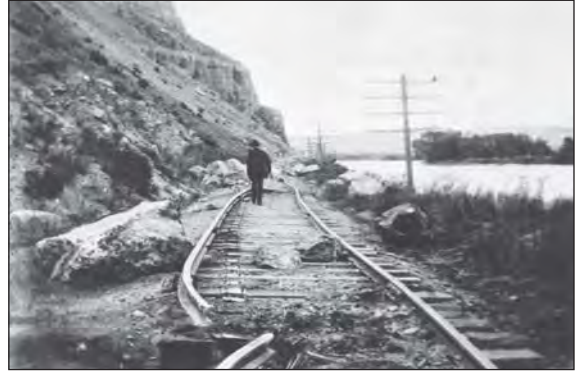
Figure 5. Broken railroad track near Lombard. Note rebound of the broken rail. Photo by J.P. Swarts. Broadwater County, Montana. 1925. Published in U.S. Geological Survey Professional Paper 147, Plate 8-A . 1927. USGS Library Image file: /htmlorg/lpb566/land/pjt01615.jpg
