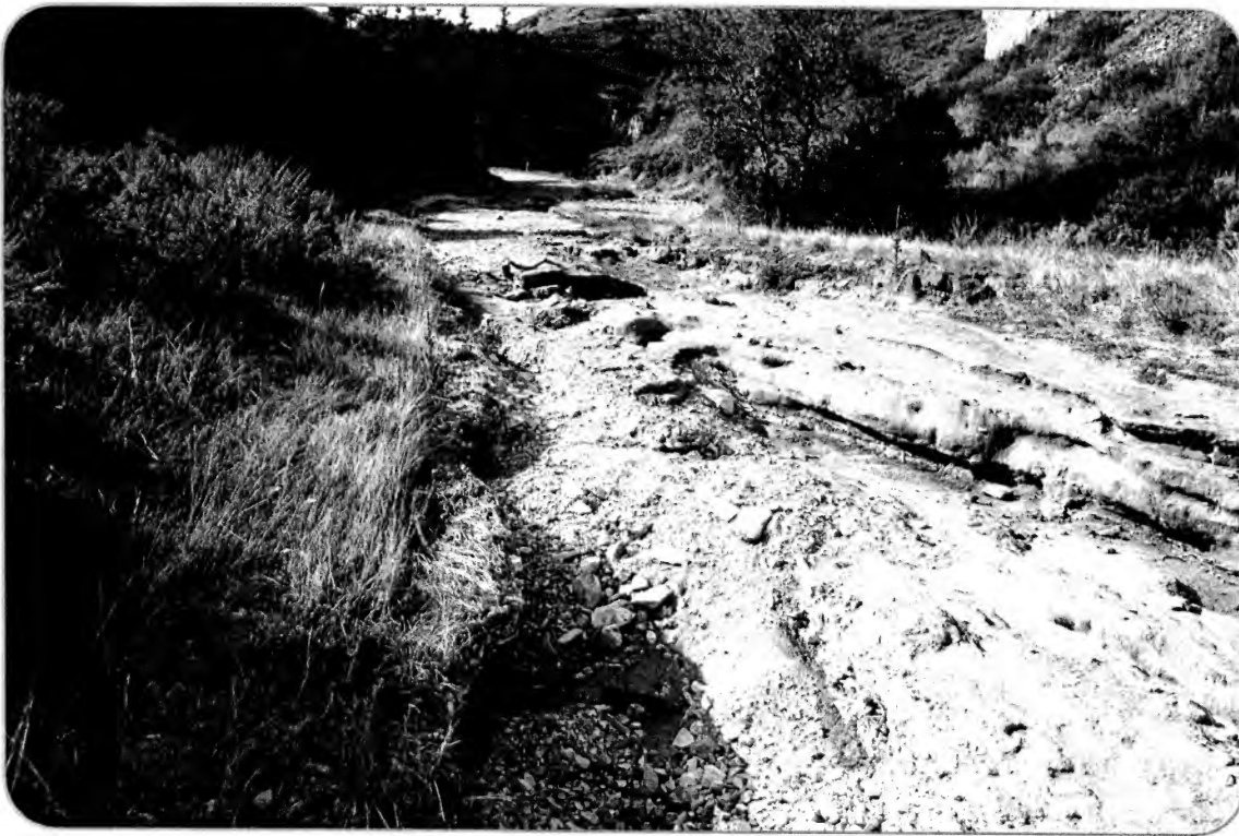
Eddies in the flood waters on July 3rd, washed out potholes in the road.
