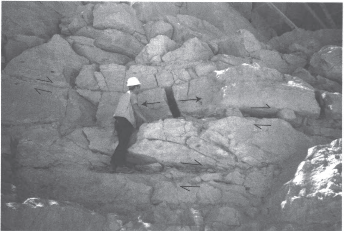
Figure 9. Open vertical to steeply dipping cooling fractures in Huckleberry Ridge Tuff offset by horizontal shear zones in the north key trench of the Teton Dam. Both sets of open joints allowed piping of water from the reservoir, which eroded the core of the dam and caused its failure. Arrows indicate relative motion along shear zones (from Embree and Hoggan, 1999, p. 188).
