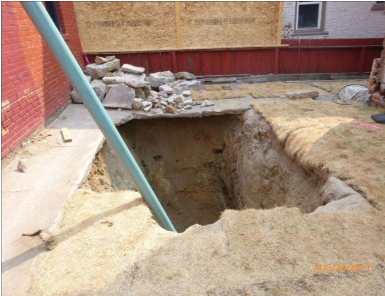
Figure 2. Sinkhole related to the Carrie Shaft (Courtesy of The Montana Standard; 2018).
