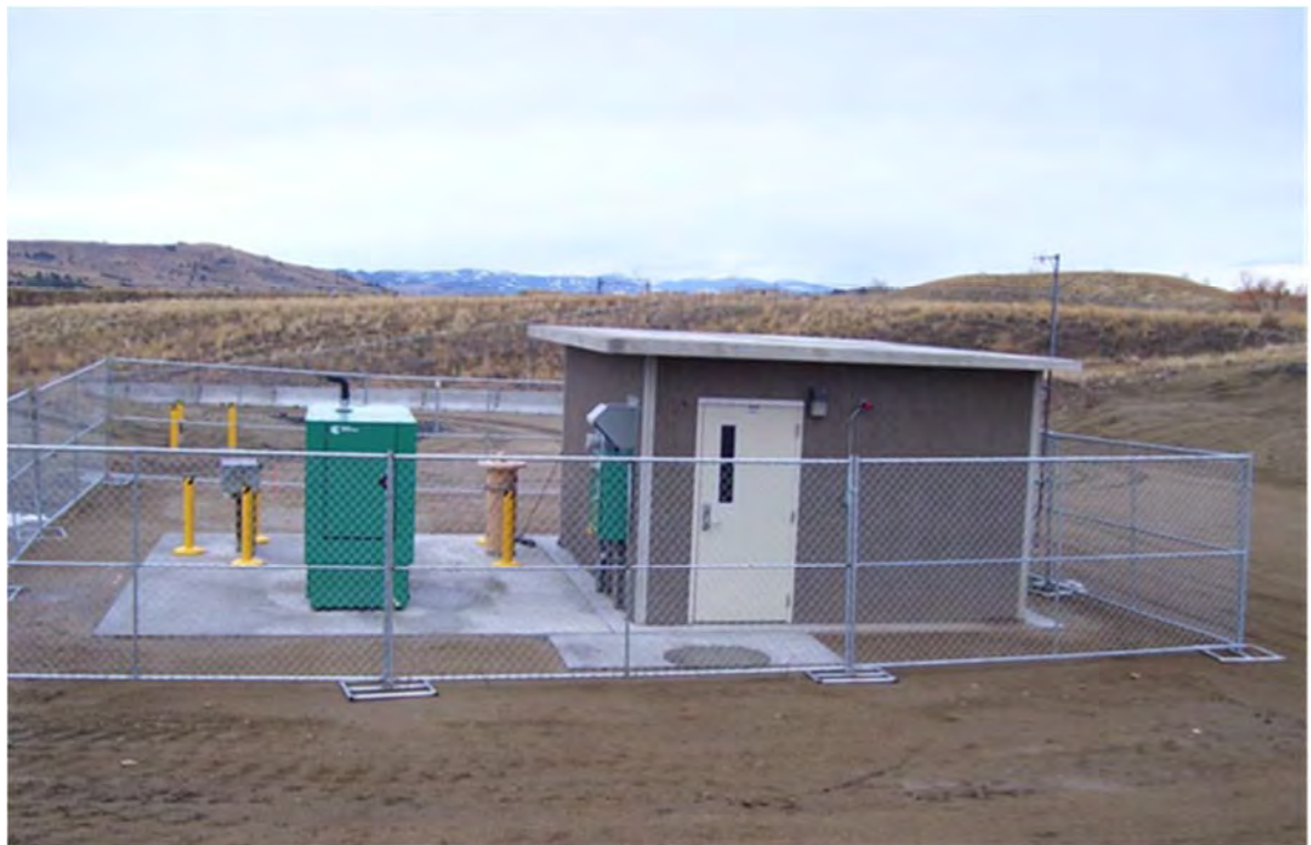
Figure 4-5. New West Camp pump station, 2011.
