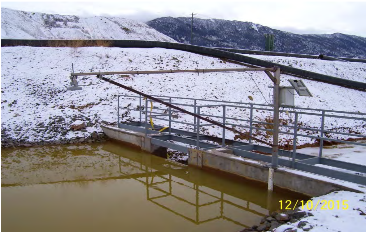
Figure 3-21. Radar system installation at the Horseshoe Bend weir monitoring station.
