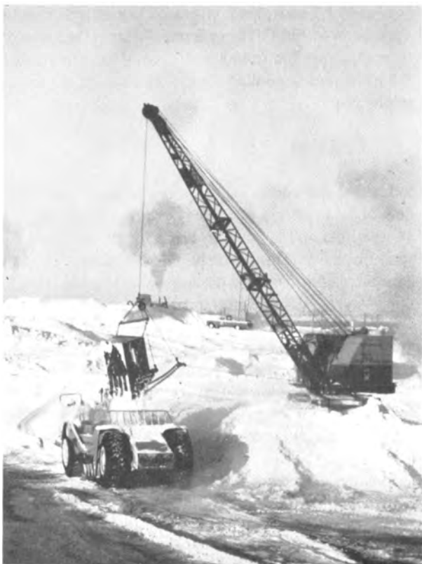
Figure 2-6.—At Chaplin Lake a dragline is utilized to harvest the salt bed that has precipitated in each of the 1,000-foot square reservoirs.
