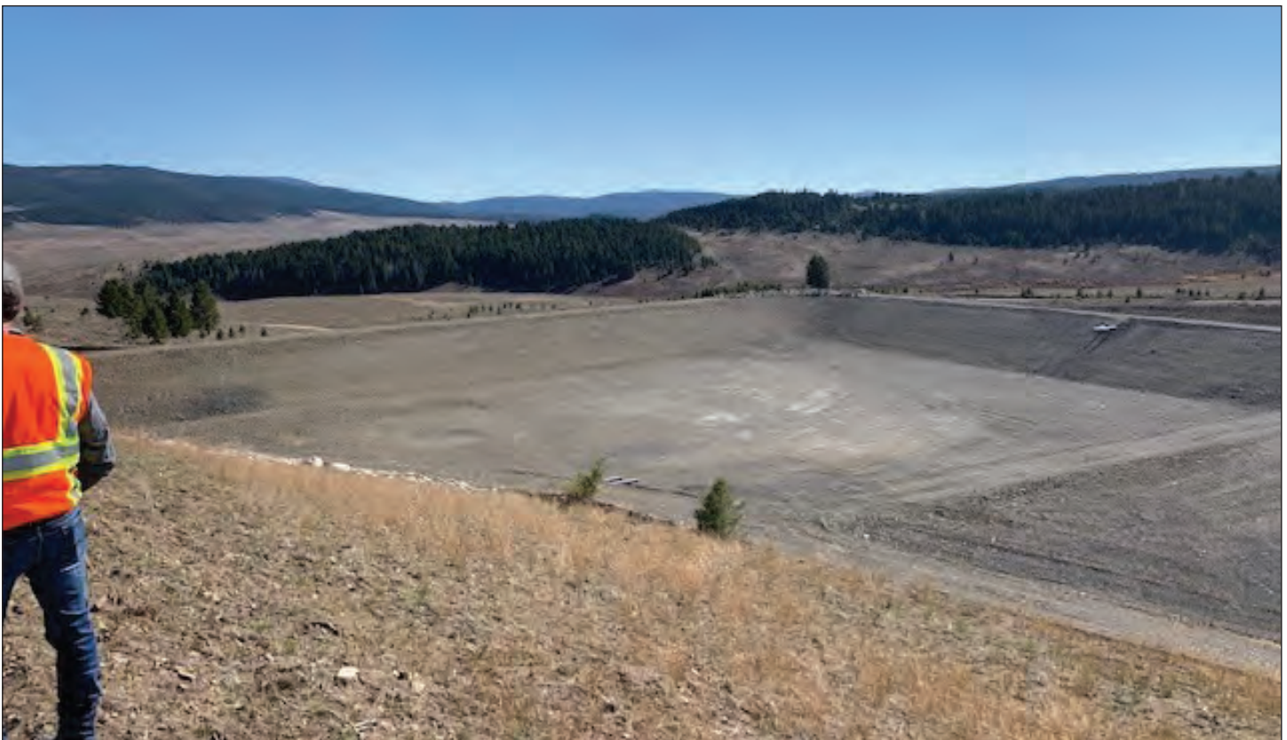
Figure 4. Phase 1 construction of the Contact Water Pond facility at Black Butte Copper.
