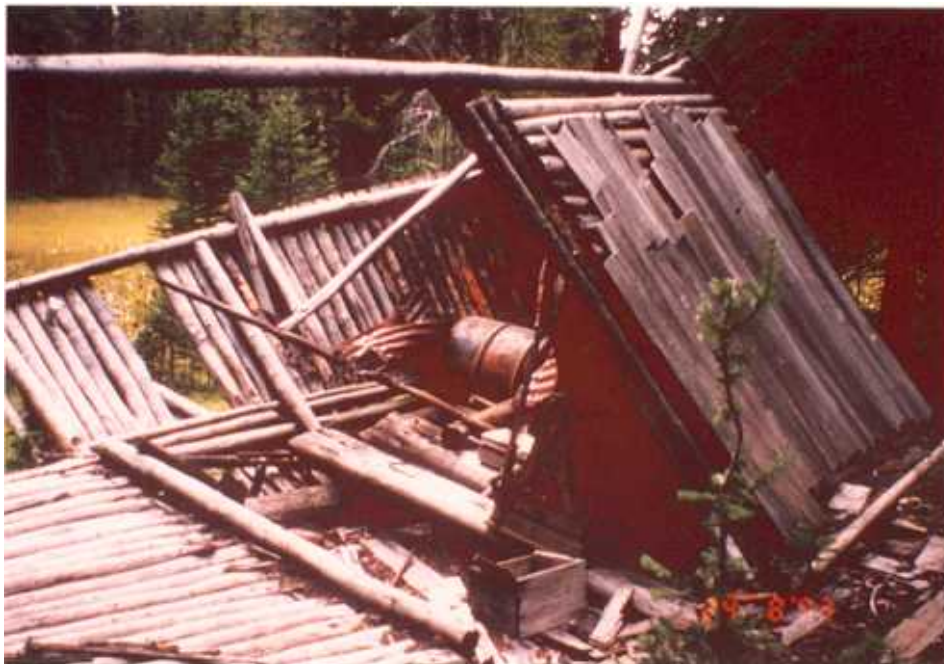
Figure 3.22 A dilapidated mine building (B-1) with some old machinery is south of shaft S-3.
