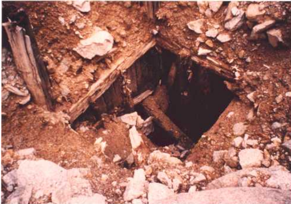
Figure 3.18 Open, flooded shaft at the Heaney mine. Depth to water is approximately ten feet.
