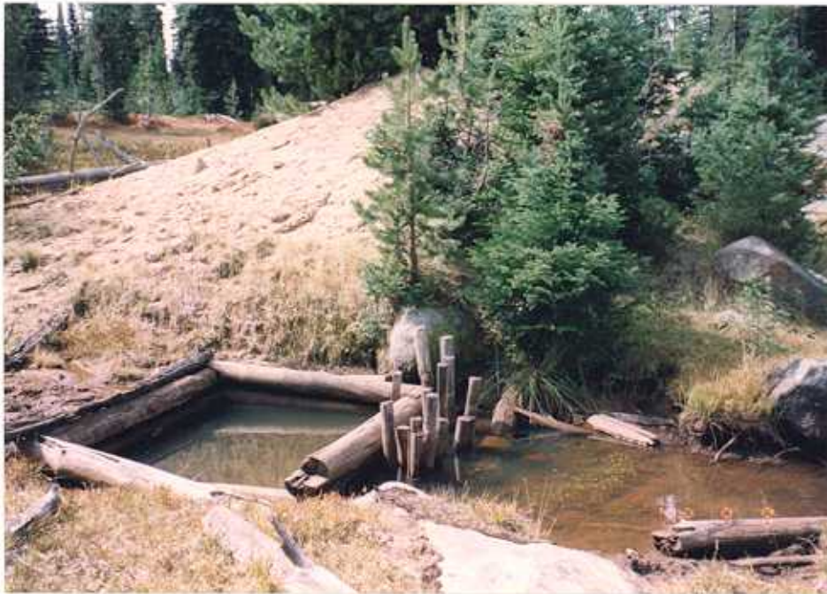
Figure 3.15 Flooded shaft S-4 has a discharge which also flows into the wetland east of the site.
