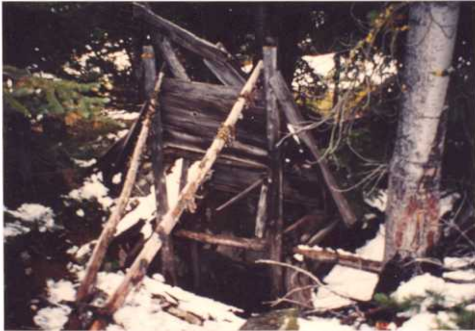
Figure 2.5a The S3 shaft at the Eldorado Mine appears to be intact.
