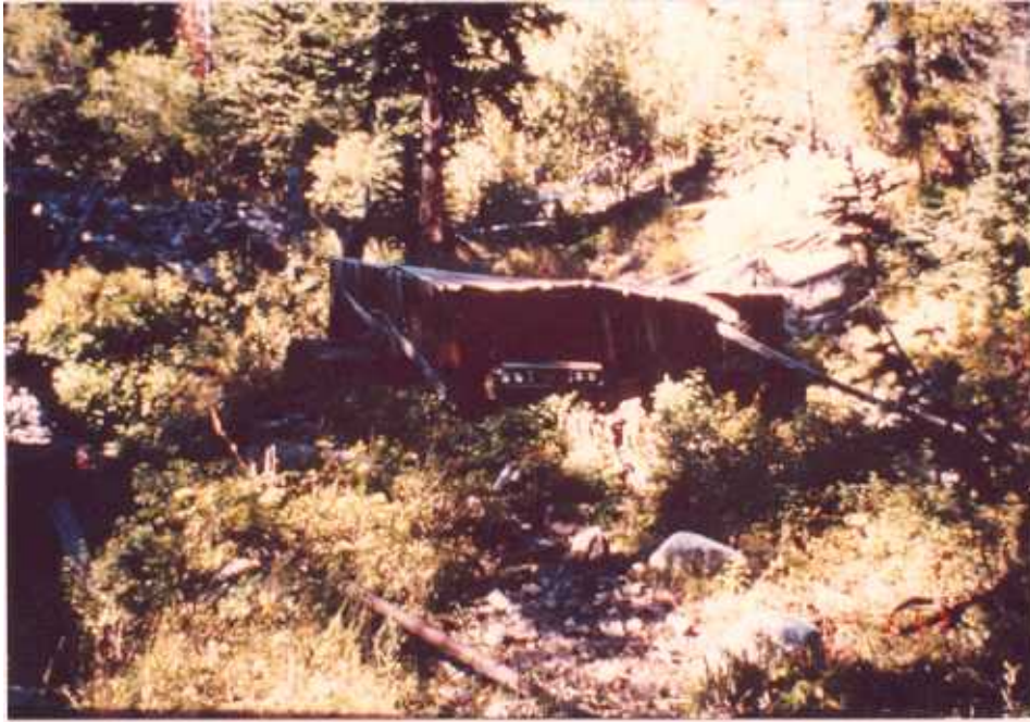
Figure 2.9a A 15-20 gpm discharge flows from a waste-rock dump south of the collapsed A2 adit and an old mine building.
