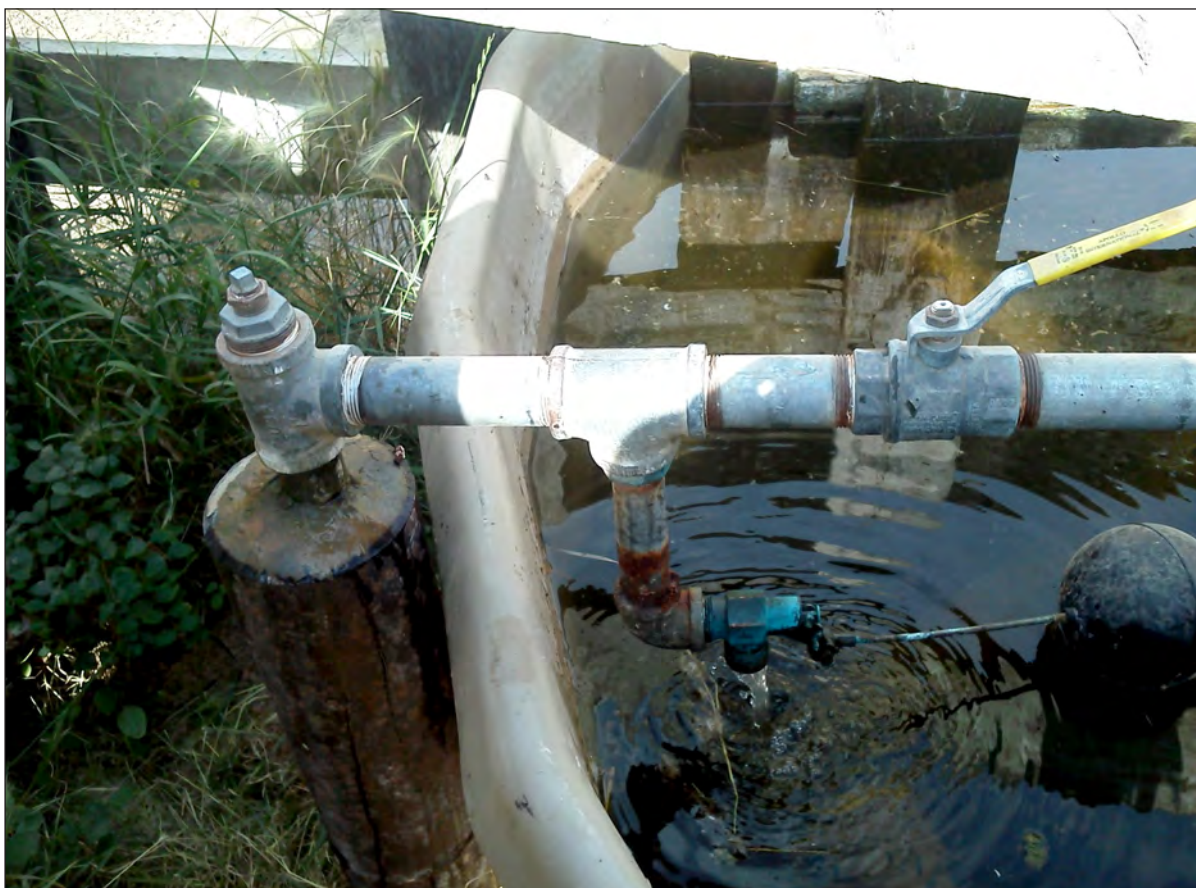
Figure 12. This tank has a control valve to shut the water off in the summer, but the valve is opened in the winter to prevent well head freezing (well 35268). The 2-in galvanized pipe casing is leaking around the cement grout.
