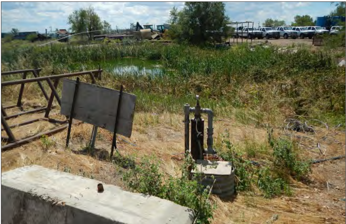
Figure 10. A wetland has formed from the overflow from the storage tank. The well head and plumbing needs to be winterized before flow could be shut during freezing conditions. (Well 35890.)
