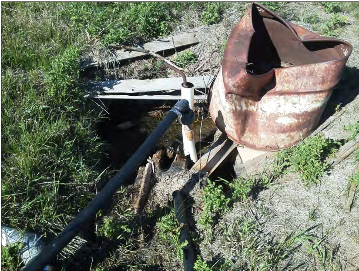
Figure 8. Leaking valves and plumbing creating erosion and a wetland at the well head.
