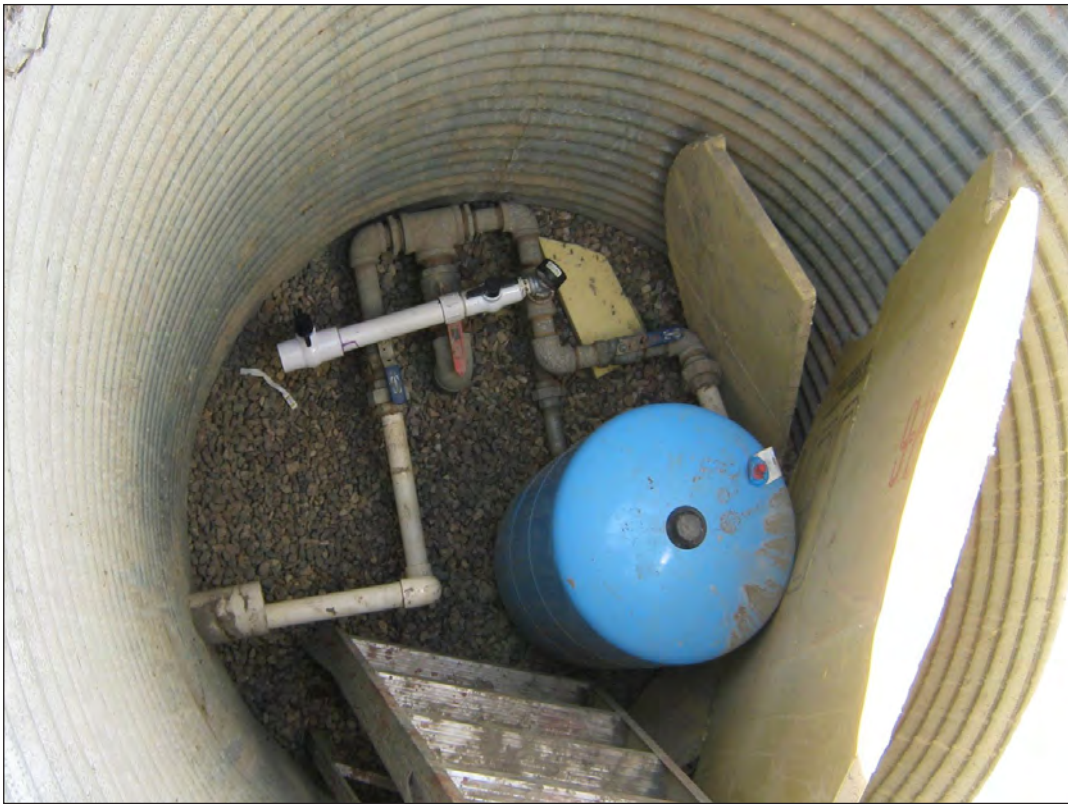
Figure 17. Well pit at well 39461 prevents well head freezing.
