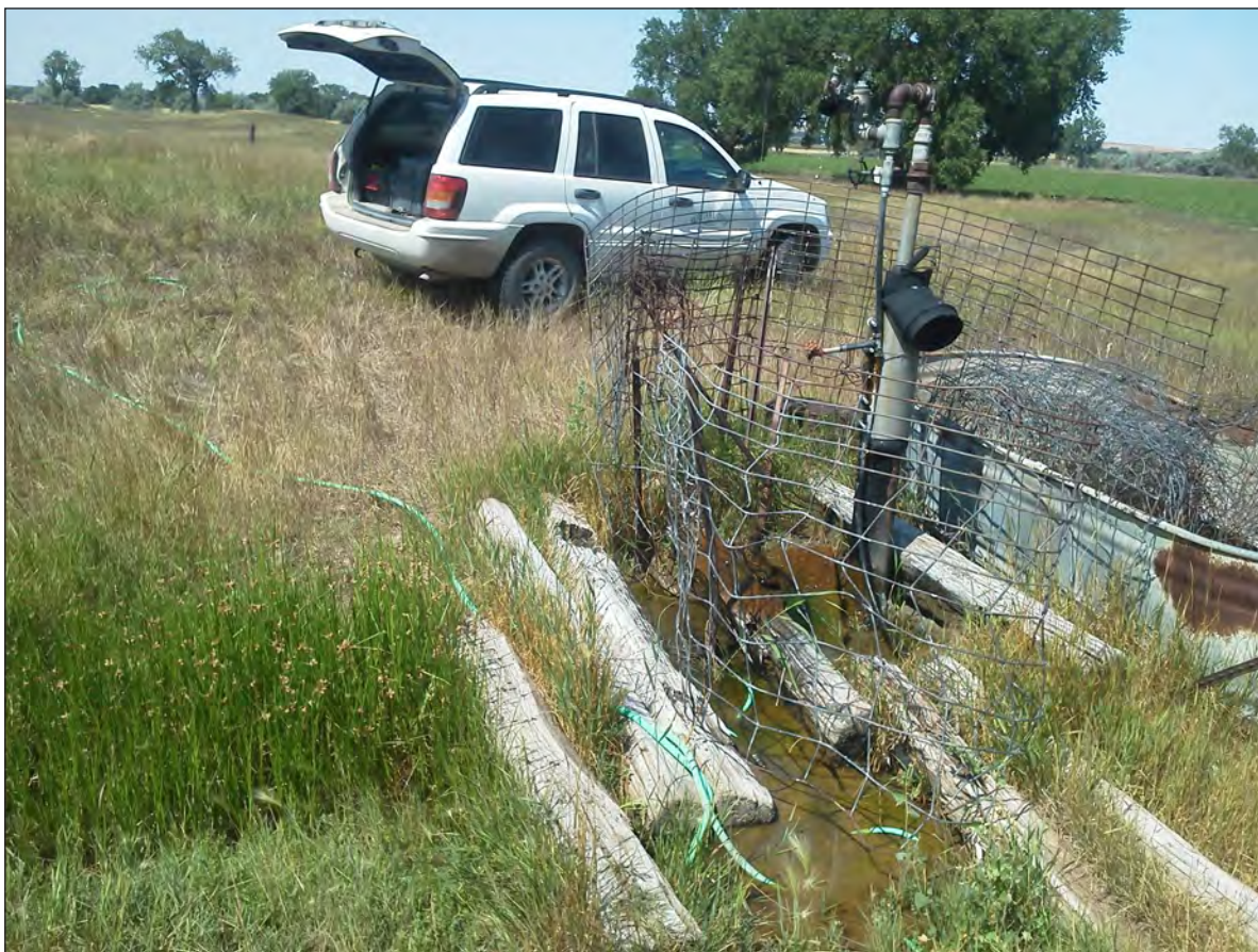
Figure 11. The surface casing (well 34259) has cracks from freezing. The casing and valves are leaking.
