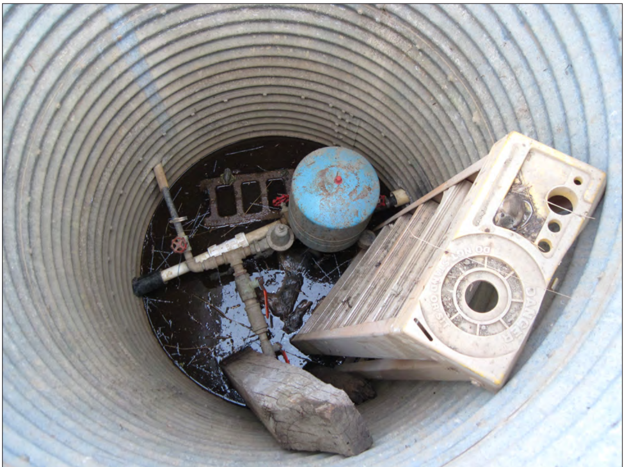
Figure 14. The well pit prevents freezing, but leaky plumbing is problematic. The pit cover is not secure, allowing animals to fall into the pit.
